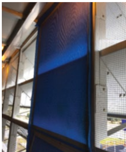
3. Blanket filter proved optimal for capturing the 2- to 5-µm particles that dominate in the inlet air at the plant location
